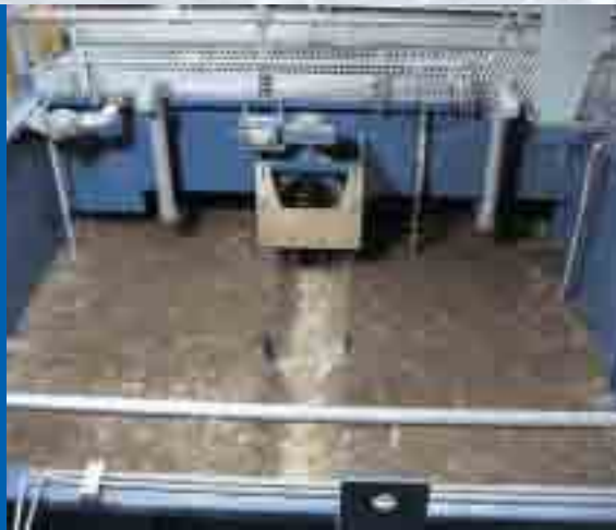
Backwash water flowing in trough, air assisted.
